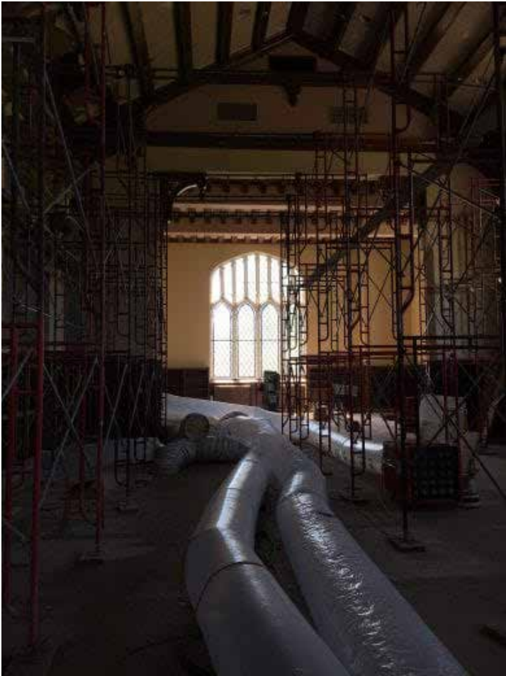
The dehumidifier tubes removing moisture from the Great Room, and a second set of tubes is pumping chilled air in.
