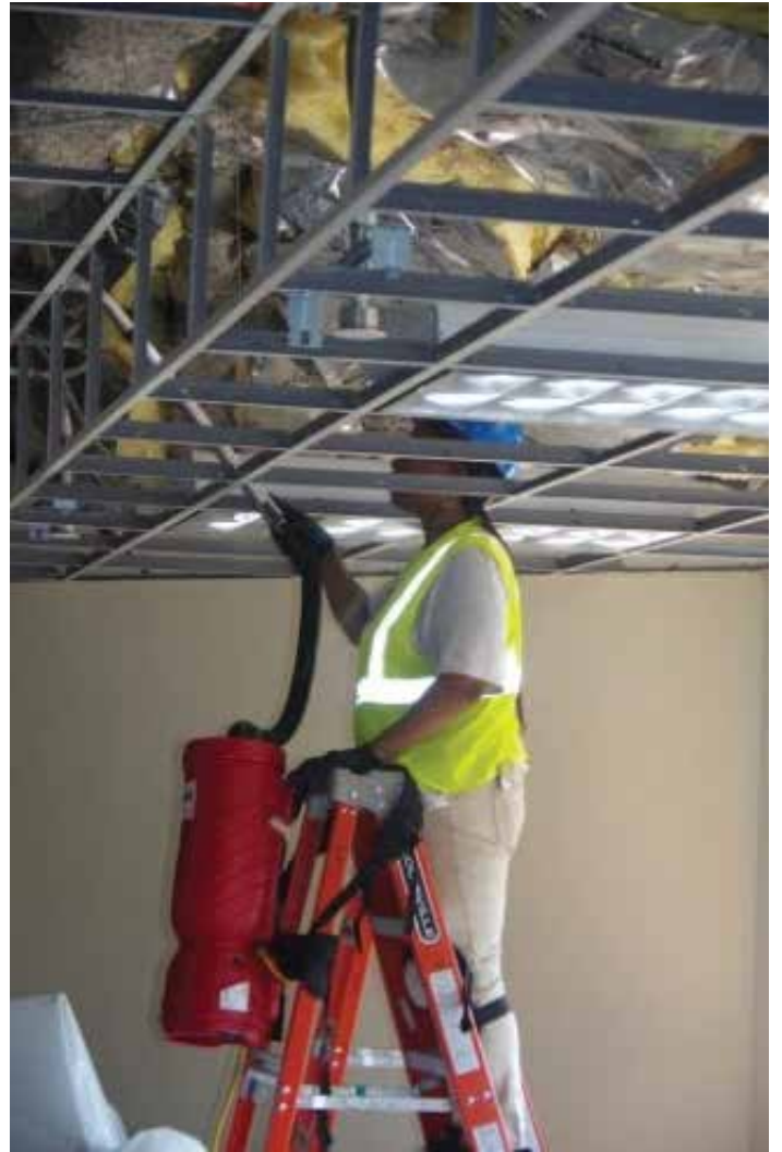
All surfaces are cleaned with HEPA vacuums before they are wiped down with chemical sponges.
