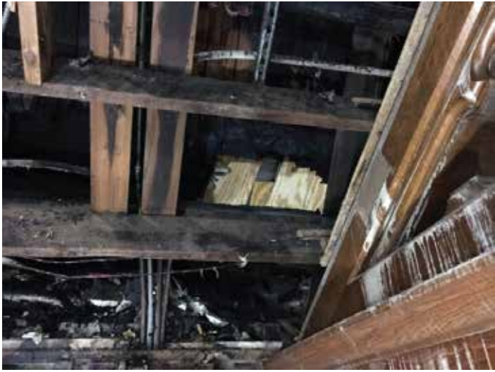
Charred, scary holes up close and personal in the ceiling that have been covered by a temporary roof.
