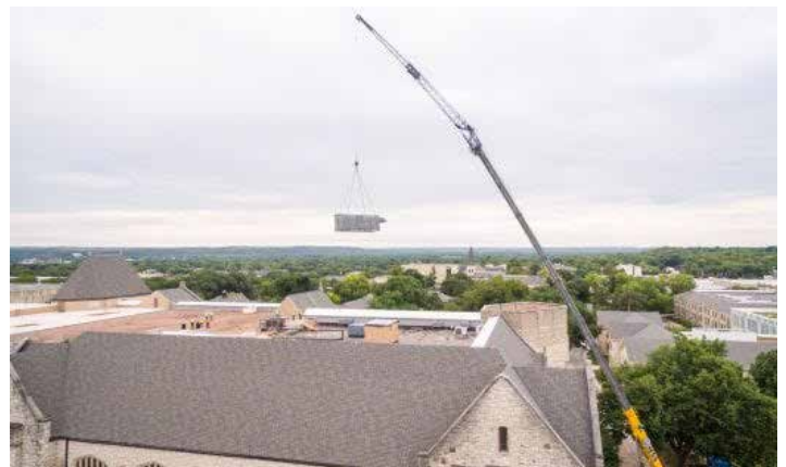
Three massive heating, ventilation and air conditioning (HVAC) units on the roof that were close to the source of the fire were deemed not salvageable, so they had to be removed.
