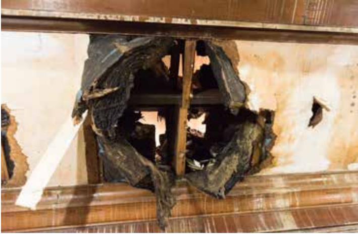
A hole in the Great Room ceiling.
