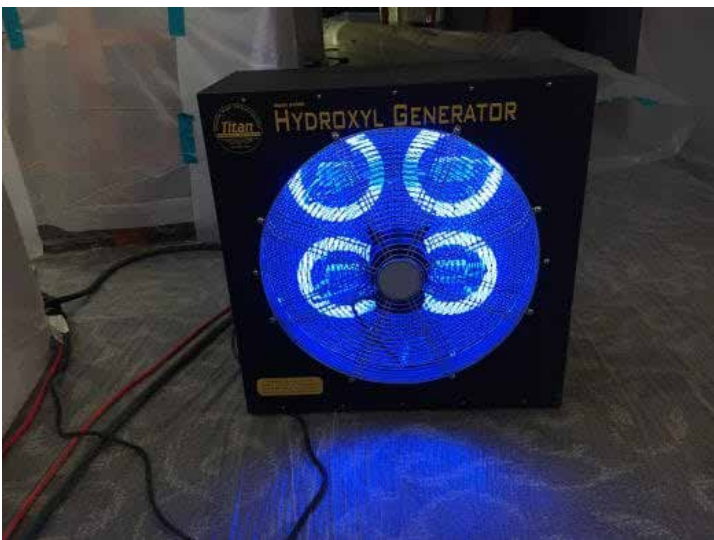
There are multiple boxes emitting an eerie blue glow across fifth floor. These hydroxyl generators use a phenomenon that occurs in nature to neutralize odor left by the fire.
