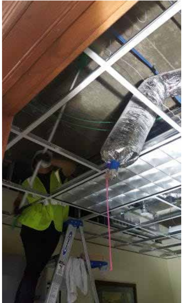
A crew member uses a chemical sponge to wipe down the ceiling and duct work.
