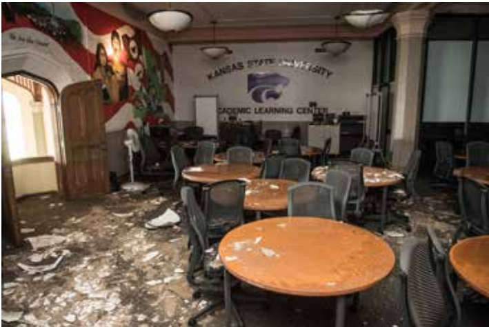
The Academic Learning Center was very near the site where the fire started on the roof and suffered extensive water damage.
