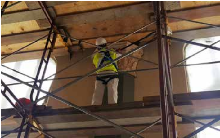
A worker removed paint from a plaster capital to allow water to evaporate from the walls more quickly.
