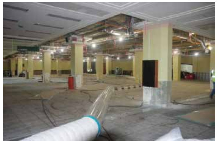
The second floor after the carpet, furniture, technology, drop ceiling system and some areas of drywall were removed.
